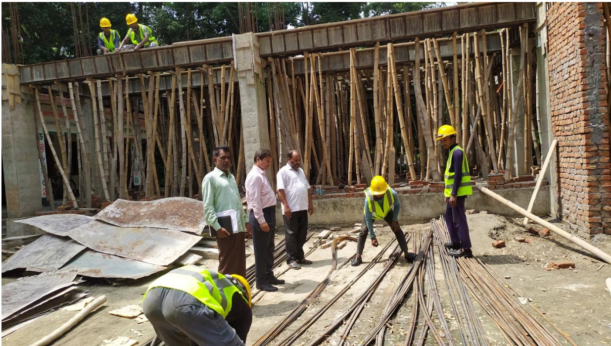
Picture: Environmental Specialist was inspecting construction works at Erulia GPS in Bogra Sadar, Bogra.
