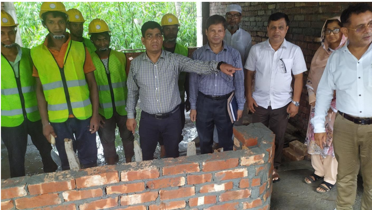
Picture: Environmental Specialist and Upazila Engineer jointly inspecting construction works at Thanthania GPS in Bogra Sadar, Bogra.
